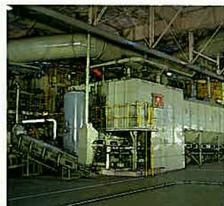
AUTOMATIC SAND TREATMENT LINE
